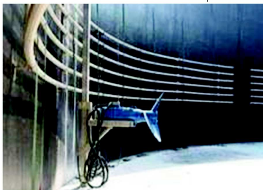
Figure 5. Small mixers (k 1 ) and installation scheme Vh – vertical setting, Hm – horizontal setting, Hs – heating tubes
