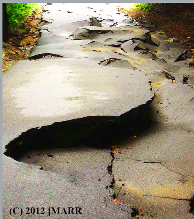
(C) 2012 jMARR May, 2012, road damage in southwest NH from storm surge runoff that destroyed culverts and roads and marooned residents for several days.
