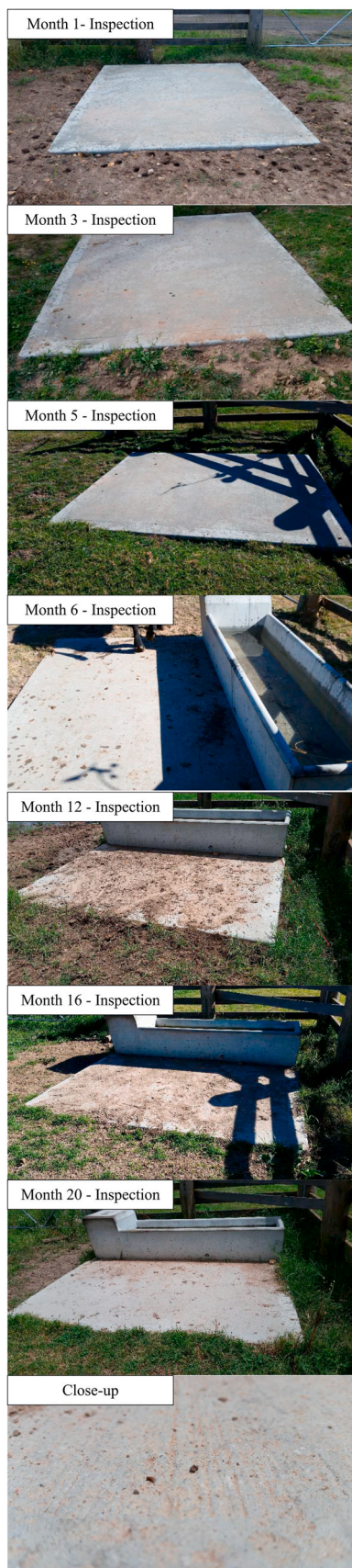
Fig. 10. 100% CO 2 Concrete slab 2 visual inspections.
