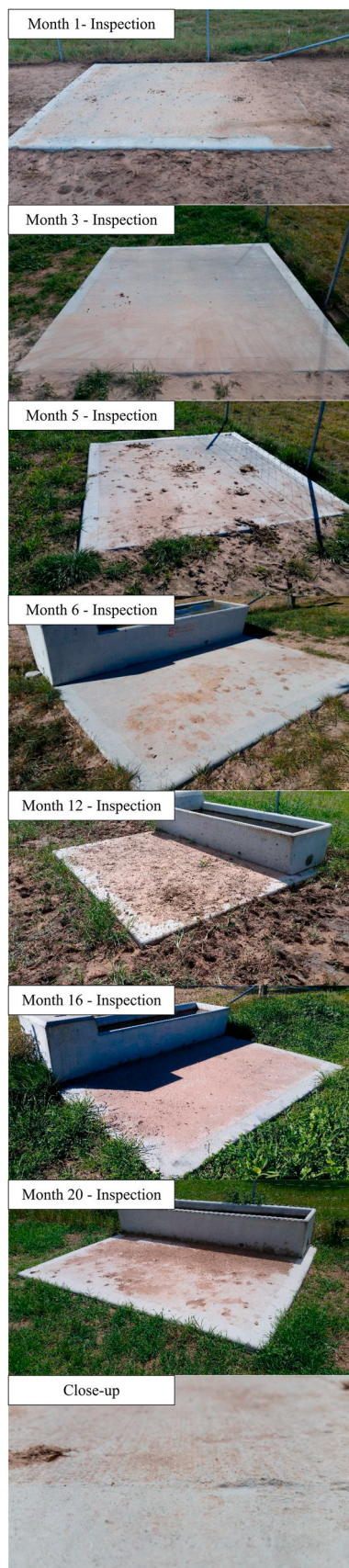
Fig. 11. 100% CO 2 Concrete slab 1 visual inspections.
