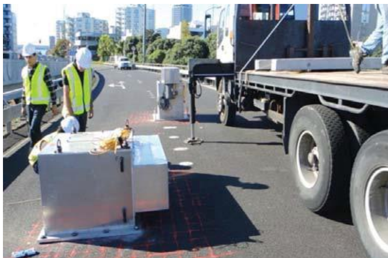
Figure 2-1: Shakers anchored to the bridge deck for forced vibration test (Chen et al. 2014)
