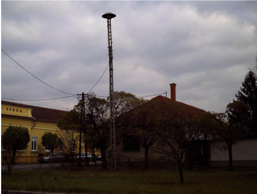
Installed residential alert terminus, disaster management powered siren Source: Szentés Civil Protection Branch
