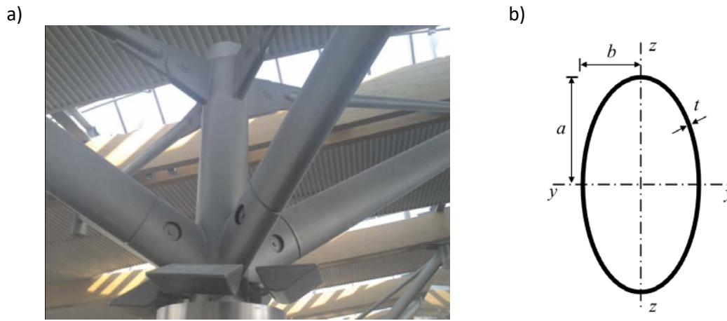
Figure 1: a) Steel EHS at Cork Airport; b) cross-sectional geometry of EHS showing dimensions and axes.
