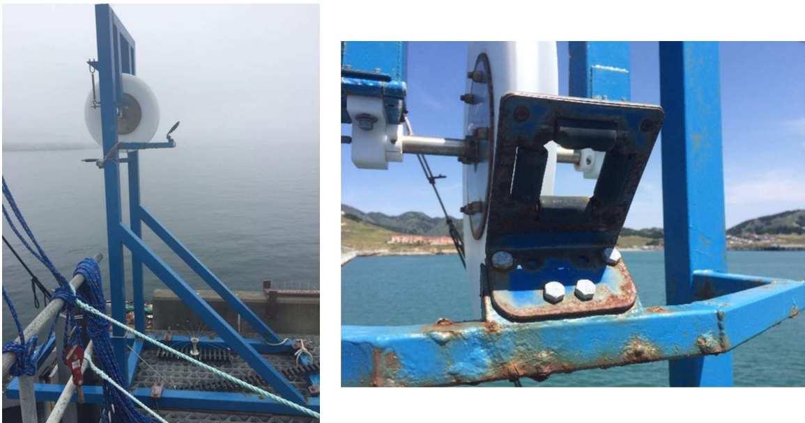
Figure 15. Original sheave holder assembly showing rust damage. (Espinosa, Pier Portal Thesis Image Repository, 2017)
