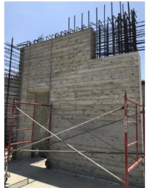
Image 3: Experimental Board Form Concrete Wall Observed on Site Visit by Dylan Thompson
