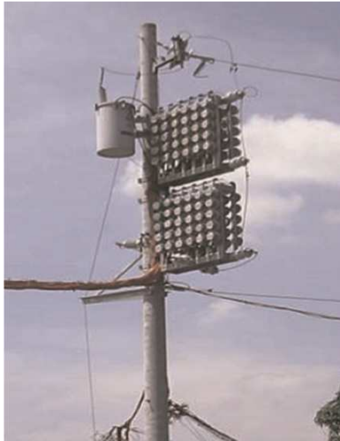
An elevated metering cluster, used to electrify informal settlements with less risk of tampering and illegality. Source: Meralco, "Delivering electricity to vulnerable communities", Asian Development Bank Asia Clean Energy Forum, June 19th 2009.
