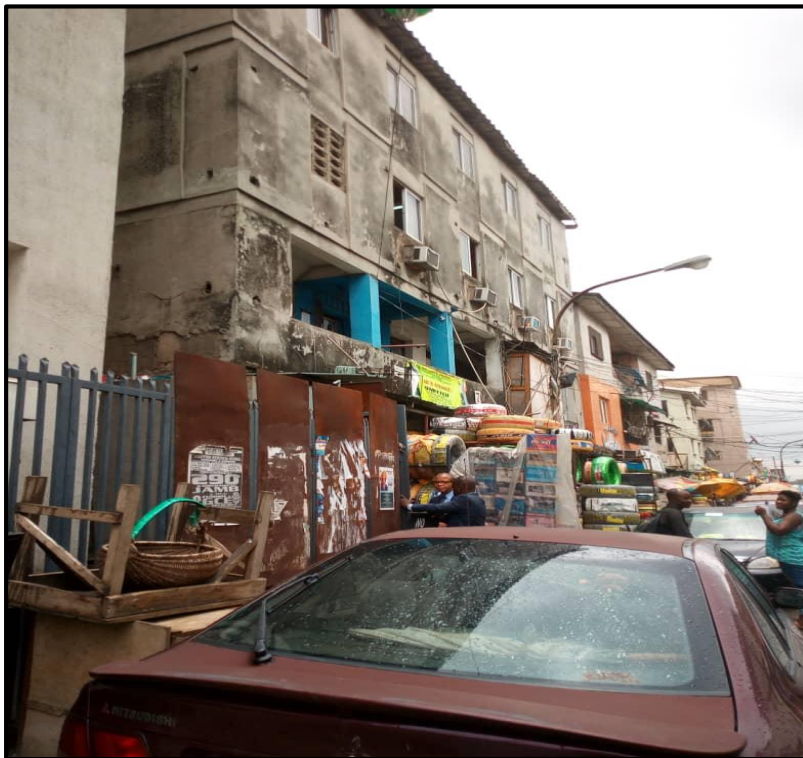
Figure 3: The effect of the climate on the plastering material on the wall of the building Source: Authors research.
