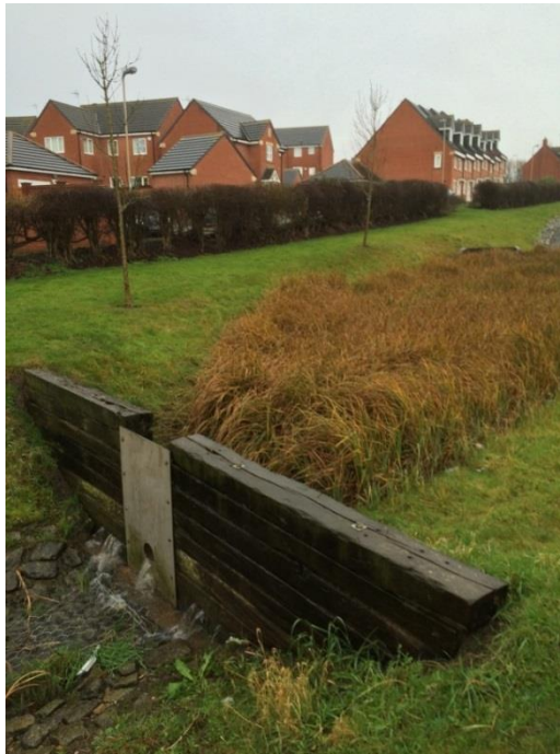
Figure 3-22 Weir 1 at start of management train, used to back up flow into the vegetated pond during large rainfall events.
