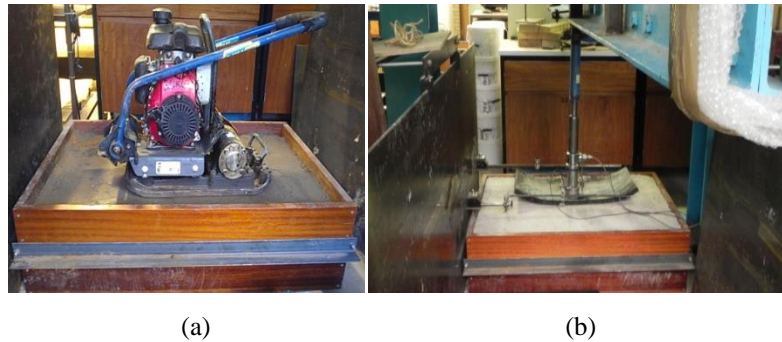
Figure 8-1 (a) cement stabilized aggregate foundation in construction; (b) overall view of loading frame
