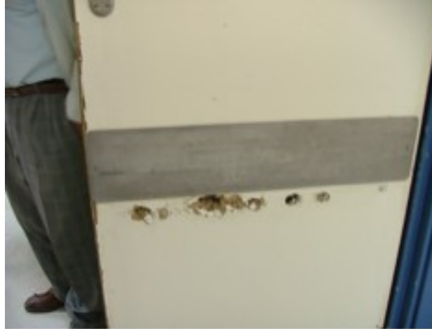
Figure 5.5: Damaged door, Düzce State Hospital.
