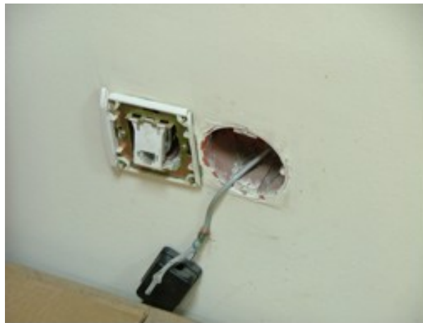
Figure 5.6: Electrical damage, Düzce State Hospital.
