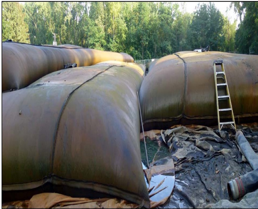
Dredged pond sediments being de-watered in large filter bags make it easier to transport the sediments to a landfill.
