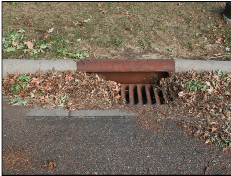
Tree leaves accumulating in a catch basin.
