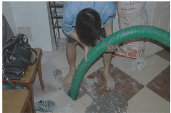
Figure 3.13 A septic tank located below a house, requiring the floor to be broken for emptying or sampling, Hanoi, Vietnam (photo: Eawag).
