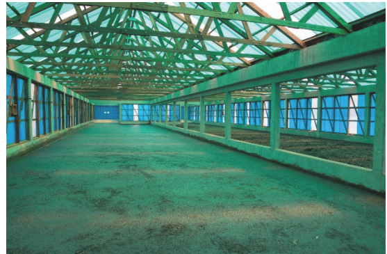
Figure 4.2 Settling-thickening tanks at Lubigi FSTP in Kampala, Uganda (photo: Eawag).
