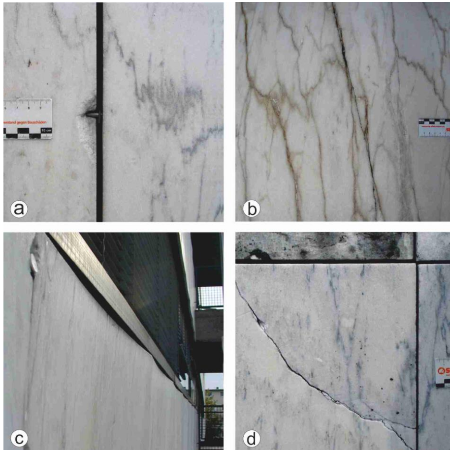
Figure 20 Damages observed in marble cladding at the State Theatre: a) outburst at a support dowel in a vertical panel joint, b) deteriorated panel with strong back weathering, c) example of concave bowing, and d) crack at a panel corner.
