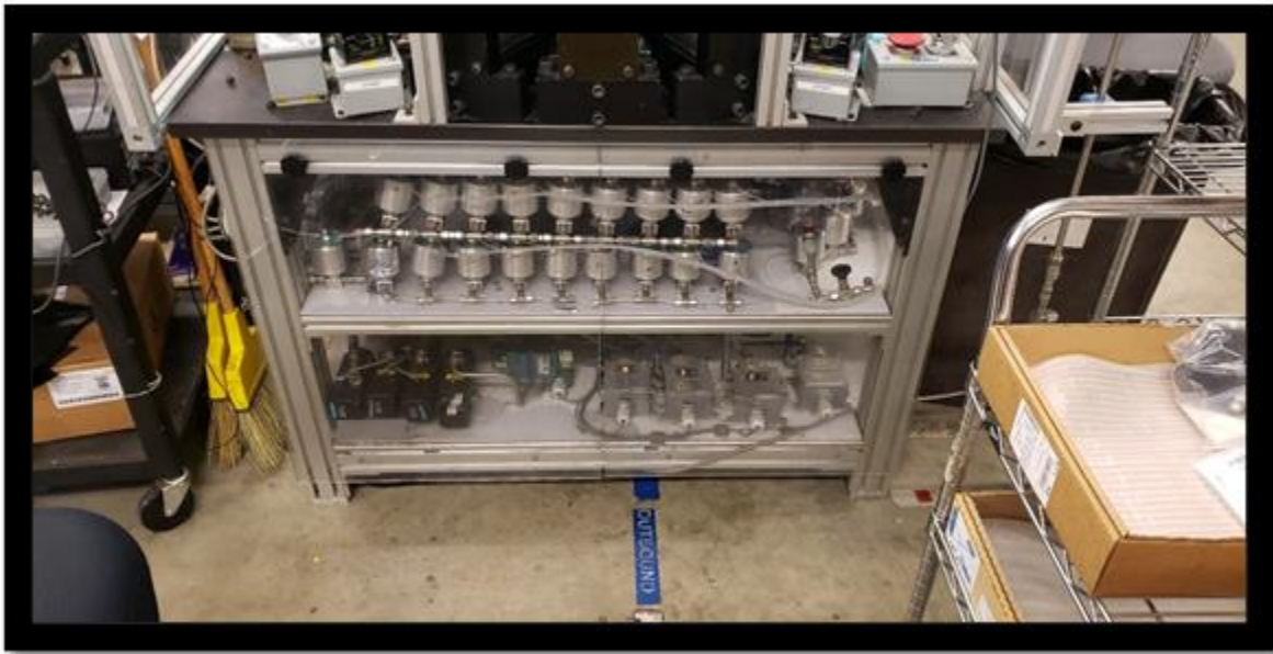
Under Table area of Tester. Note the large valve array and actuator bank with controllers.
