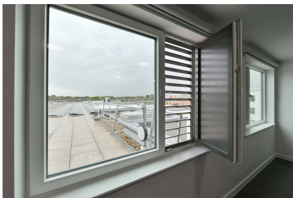
Figure 6.1: Example photo of PBSA window with louvres that would increase the opening area, while meeting health and safety requirements (LABM, 2020).
