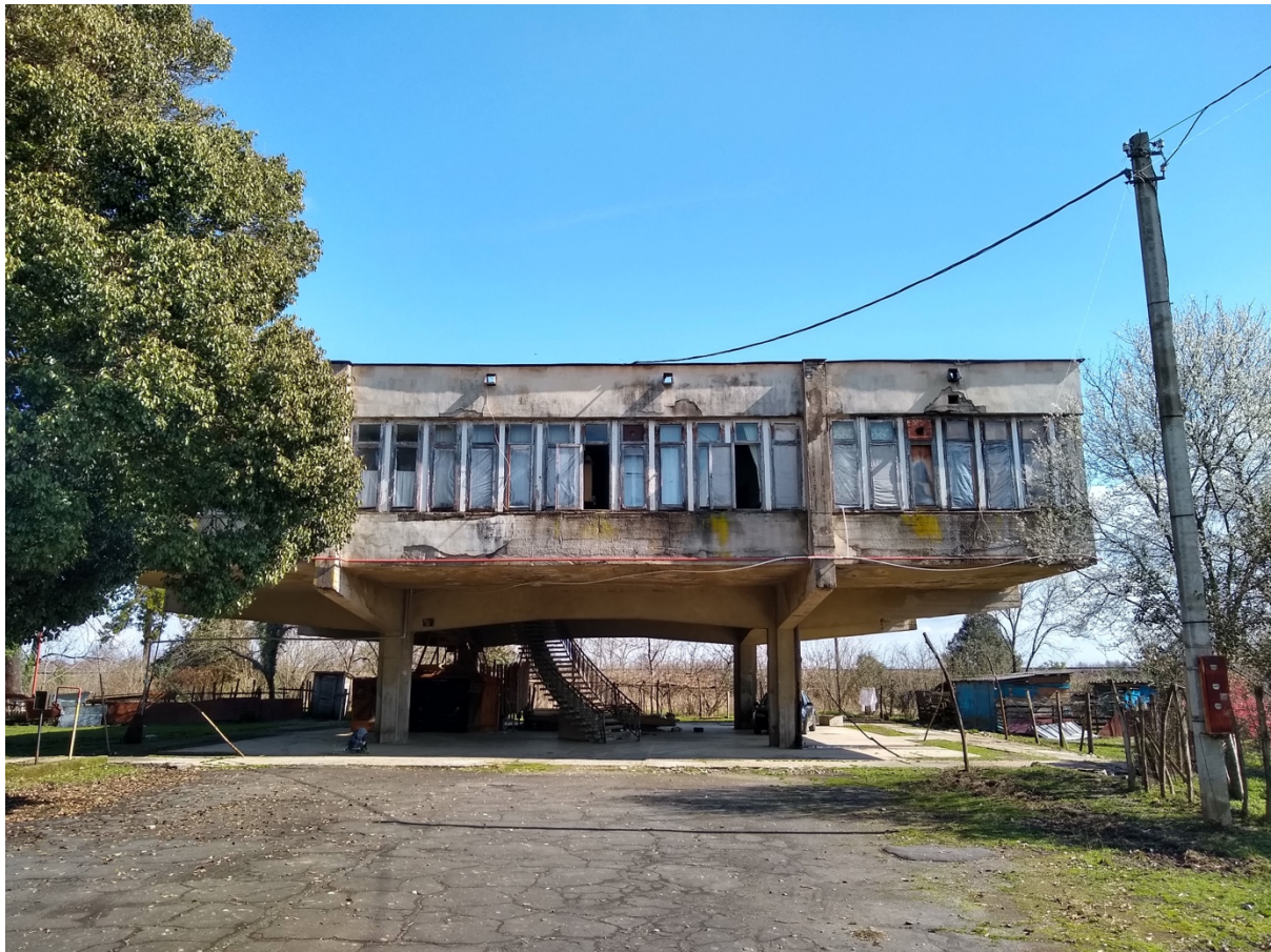
Figure 33 Former Guesthouse for the tea plantation of Ergeta, now abandoned and occupied by internally displaced people (IDP) from Abkhazia
