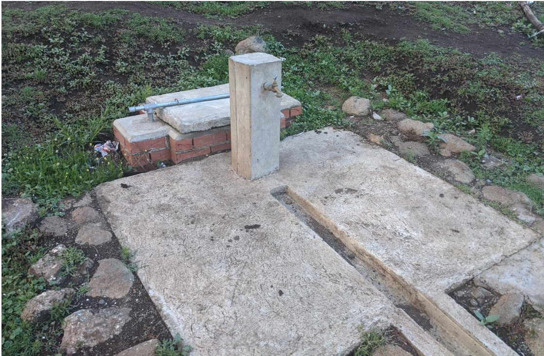
Figure 12: Photo of Village Tap 5 taken December 2019 (photo by author)
