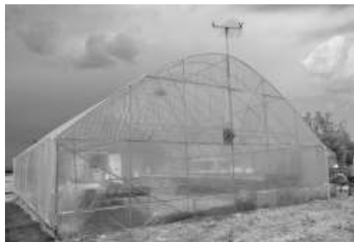
Figure 5 Wind sensors installation in a greenhouse
