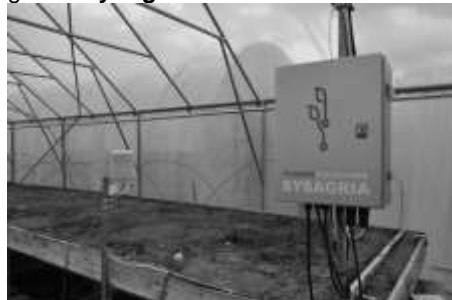
Figure 3 SysAgria cabinet installed in a greenhouse
