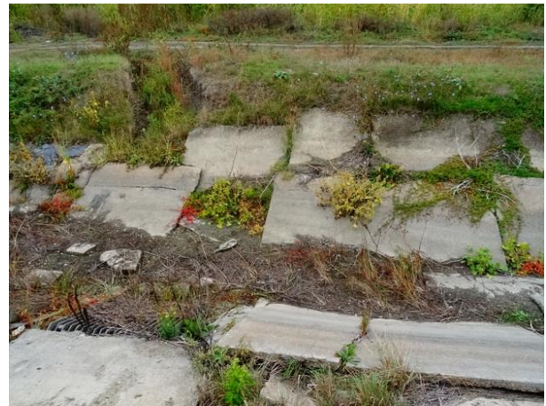
Figure 3 The state of degradation of the canals in the SPP Irrigation Plot 8 Oțetoaia with factors to increase water losses (Luca M., 2020)
