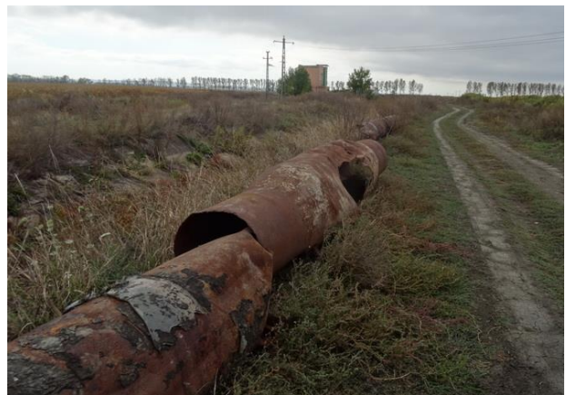
Figure 4 Degradation status of the main steel pipes in the SPP Irrigation Plot 8 Oțetoaia with water loss increase factors (Luca M., 2020)
