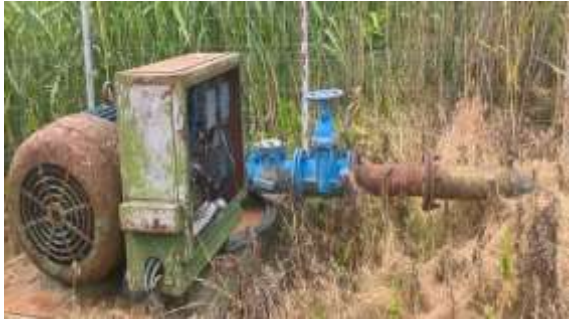
Figure 3 View of 7/5-2 pumping unit (6NDS), electric panel and discharge pipe of the SPPM 7/5 (Photo Luca M., 2016)
