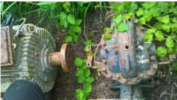
Figure 4 SPPM 7/7-2 pump aggregates status (RDN 200-150-200 pump and motor) (Photo Luca M., 2016)
