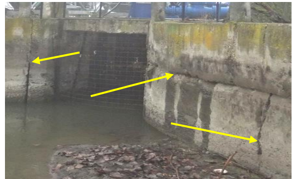
Figure 4 SPP1b Berezeni pumping plant infrastructure degradation state (Luca M., 2015)
