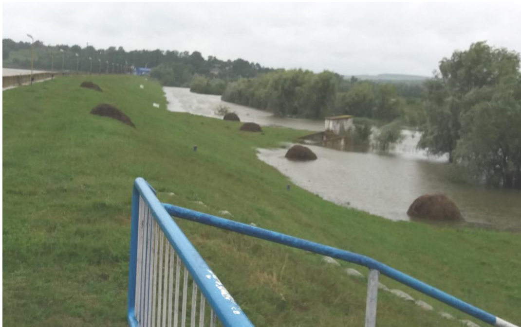
Figure 6 Dracsani dam – inundated downstream slope
