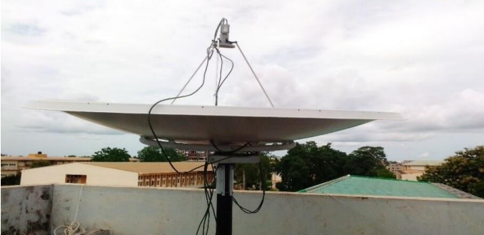
GCRF African SWIFT satellite dish installed and in use at KNUST, Kumasi, Ghana
