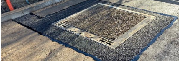
Fig. 1. A photograph of an installed wireless charging GA with approved roadway restoration completed and ready. Credit: char.gy
