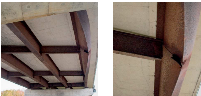
Fig. 1. Impact on girders (Photo: Edouard Berton)
