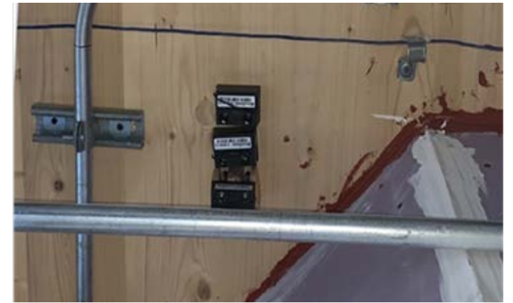
A cluster of three sensors installed in Adohi Hall to measure moisture levels. (Photo courtesy of Tahar Messadi)
