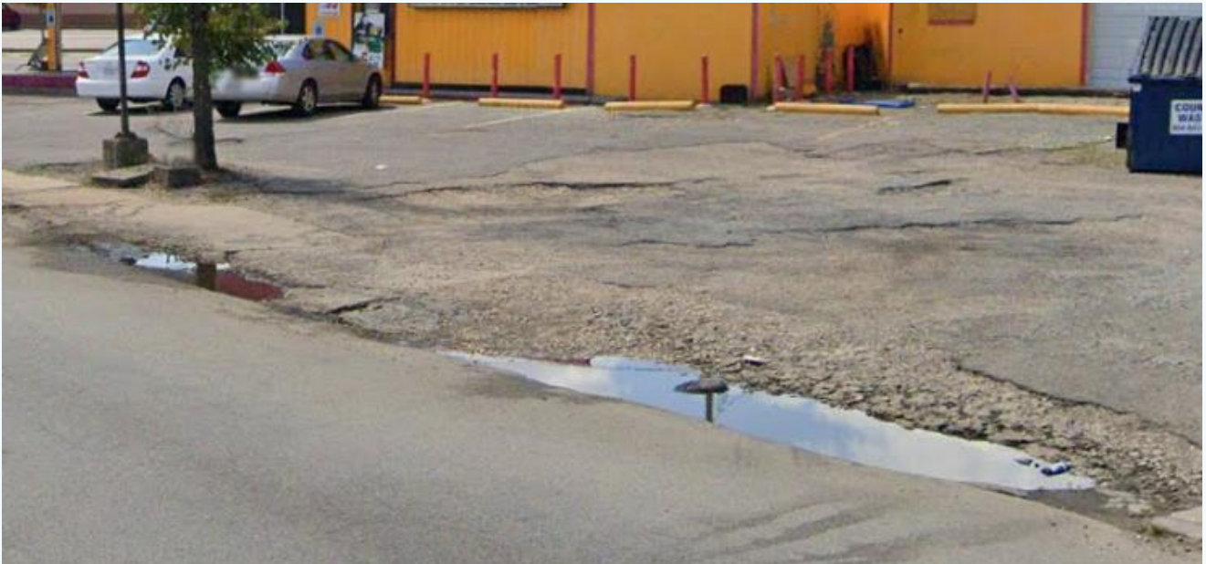
Figure 19. Sidewalk Conditions at Nine Mile Rd. & N. 31 st St.; Source: Google Maps, 2019
