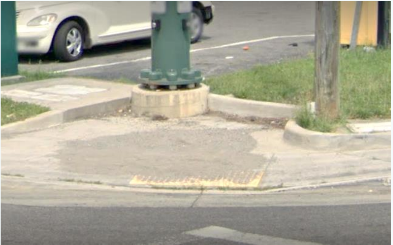
Figure 22. Worn Down Tactile Landing Surface; Source: Google Maps, 2019
