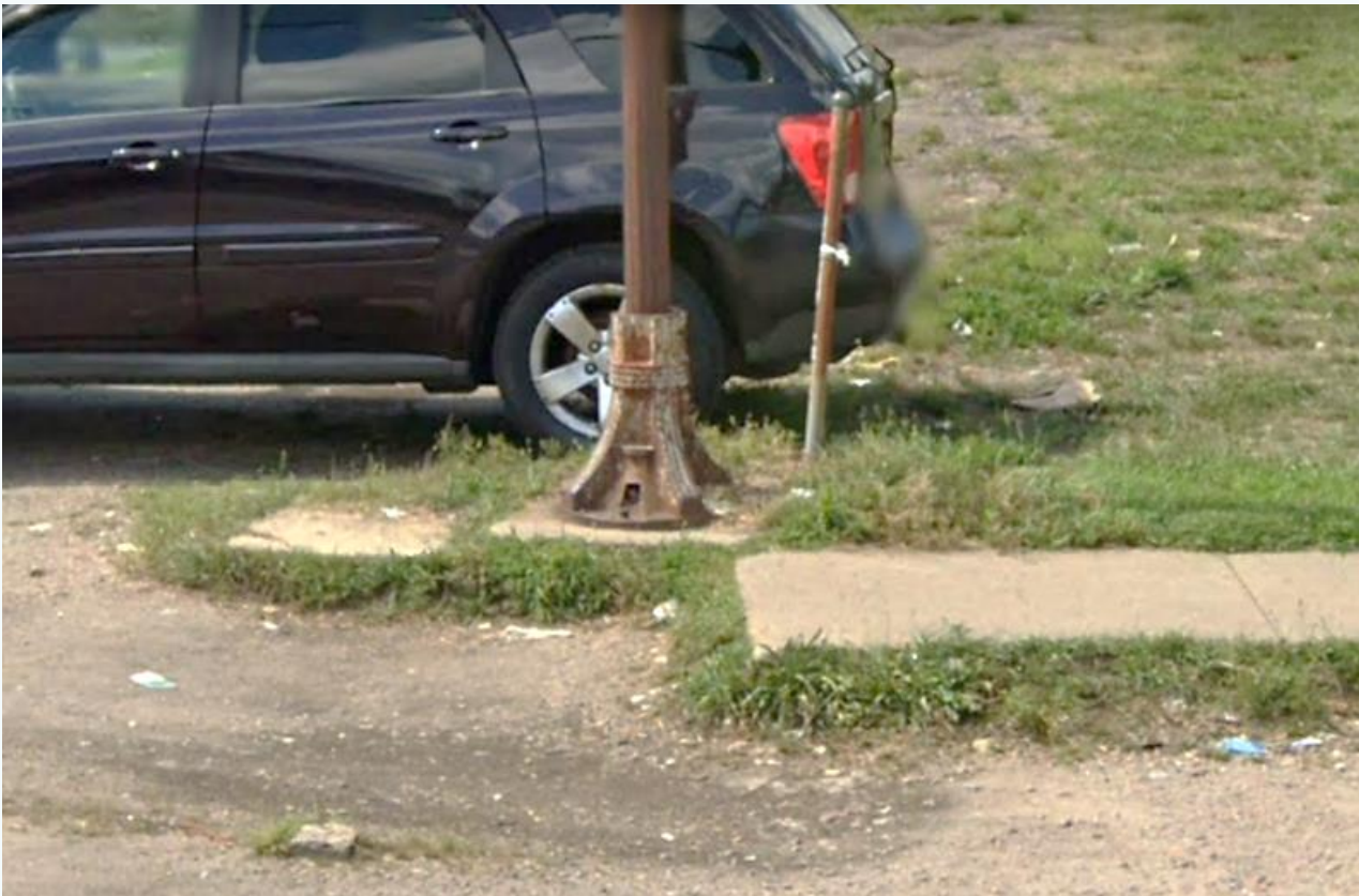
Figure 25. Inaccessible and Unsafe Sidewalk; Source: Google Maps, 2019
