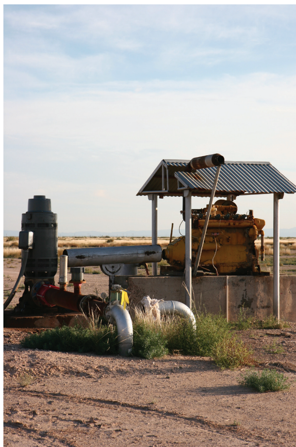
Irrigation well near Pecos, Texas
