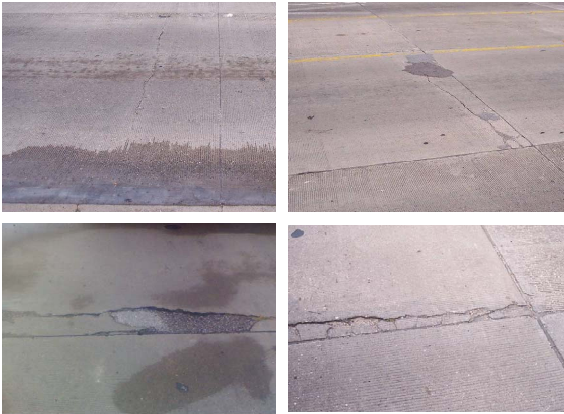
Figure 3-21 Surface Conditions of Sampled Section on FM 364.
