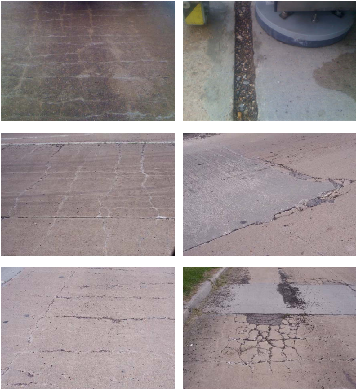
Figure 3-26 Surface Conditions of Sampled Section on IH 10.
