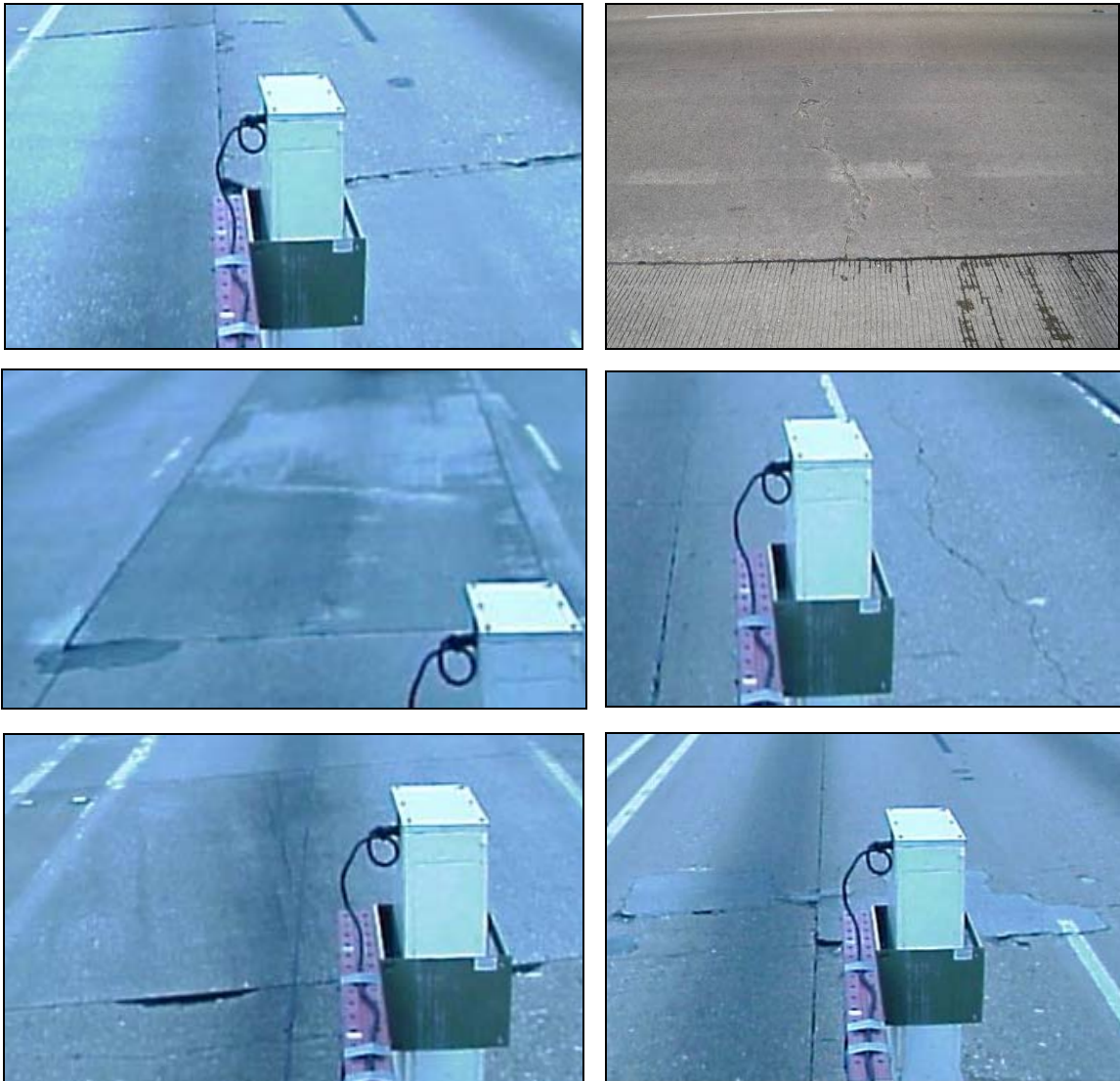
Figure 3-31 Surface Condition of Sampled Section on IH 635.
