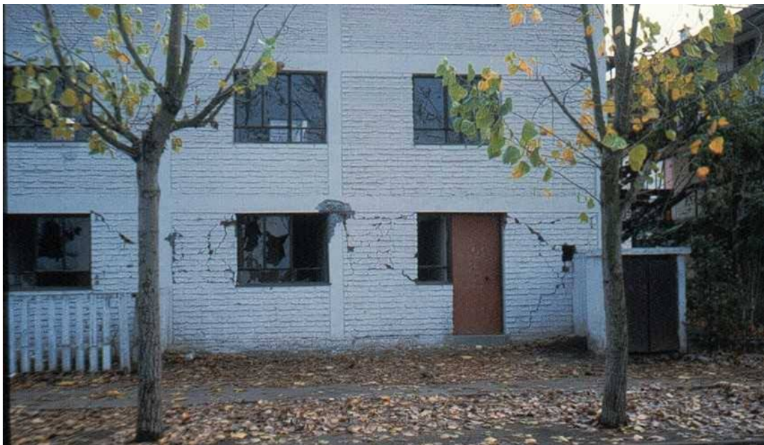
Fig. 5. Three-story partially confined masonry building; Melipilla, Chile, on March 3, 1985
