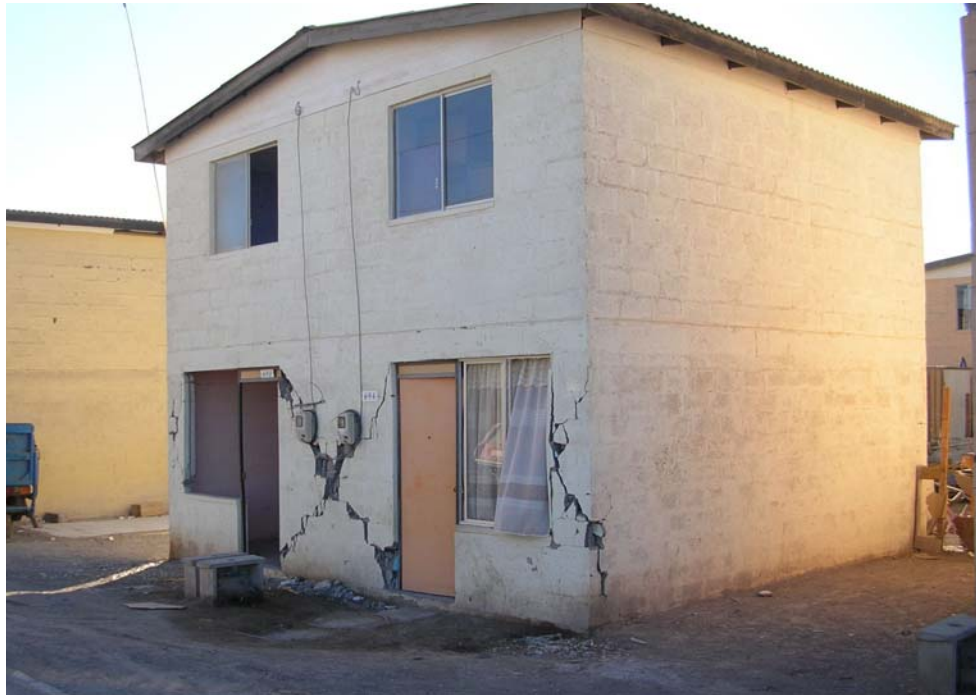
Fig. 6. Masonry house at Huará, Chile, after Tarapacá earthquake on June 13, 2005
