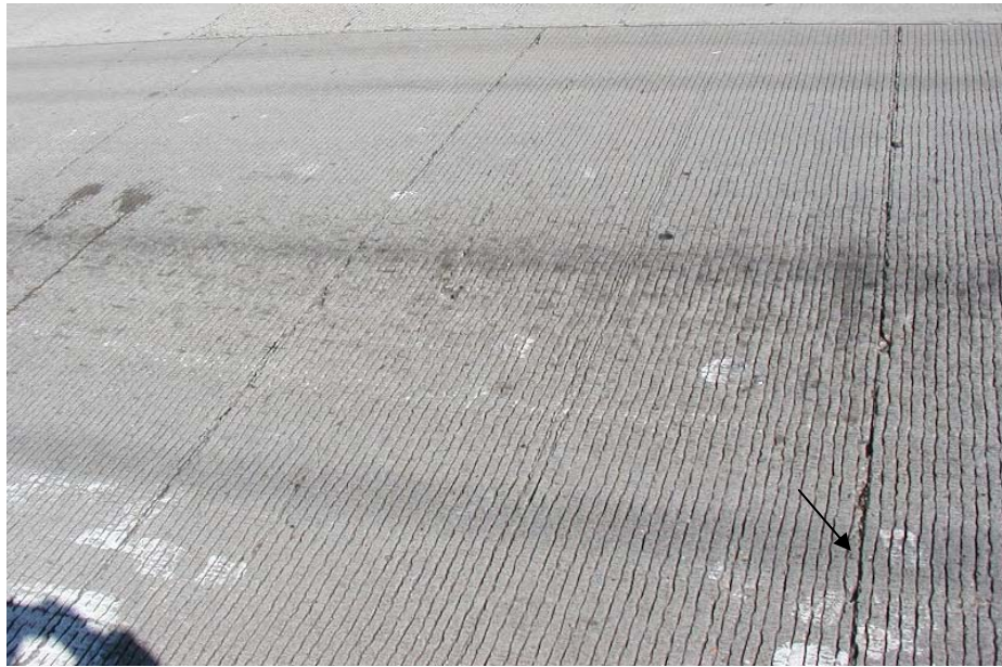
Figure 6.4 The pavement section with sawcuts before the core was taken (the arrow shows the location where the core was taken)
