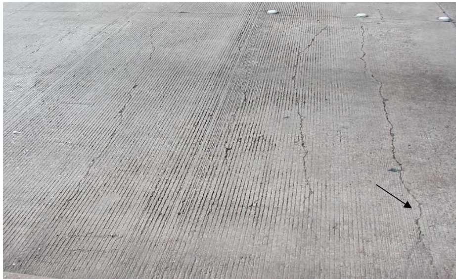
Figure 6.3 The pavement section without sawcuts before the core was taken (the arrow shows the location where the core was taken)
