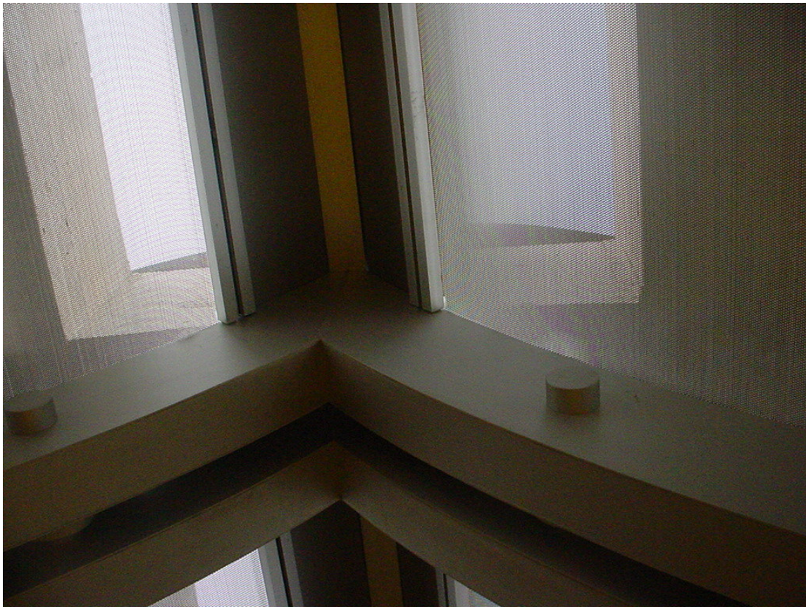
Figure 24: Detail of the perforated aluminum reflector and the slit at the apex of the vault. (Photo courtesy of M.M.H. Alnuaimi, 2005)
