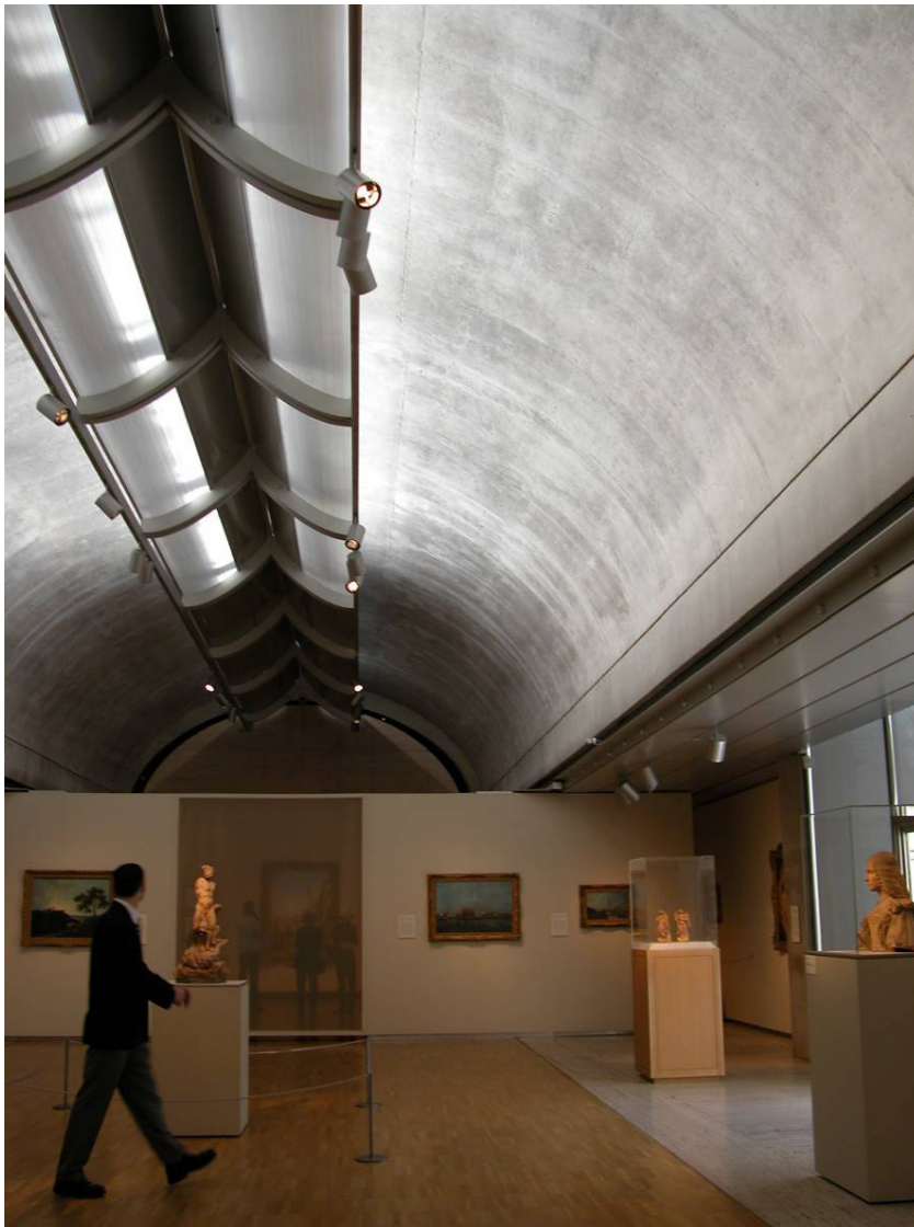
Figure 29: Interior view showing the different surface colors visible inside the gallery. (Photo courtesy of M.M.H. Alnuaimi, 2005)
