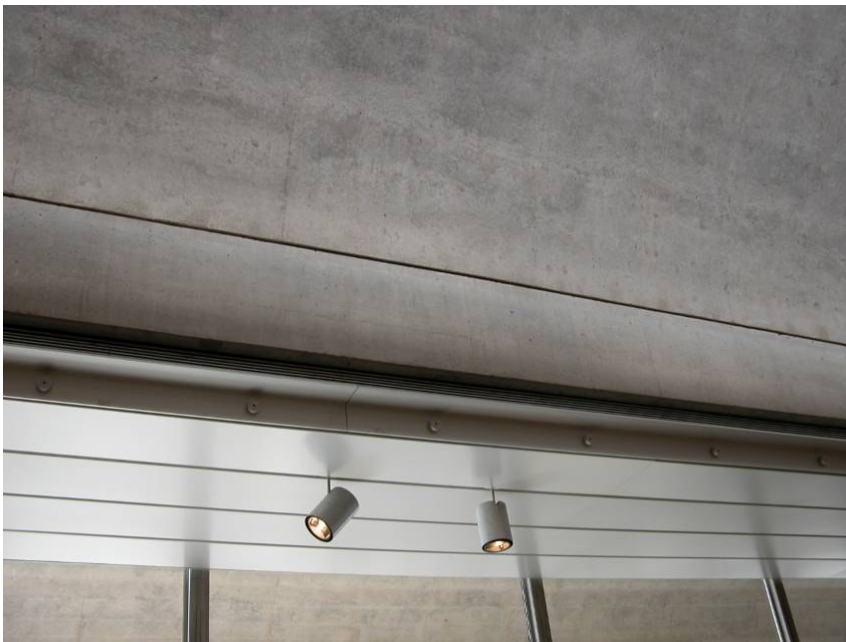
Figure 32: The 7' reinforced concrete channels with the aluminum soffits. (Photo courtesy of M.M.H. Alnuaimi, 2005)
