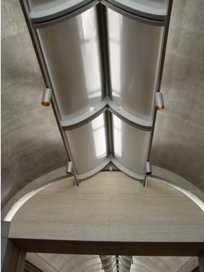
Figure 23: Detail at the gable end of the vault. (Photo courtesy of M.M.H. Alnuaimi, 2005)
