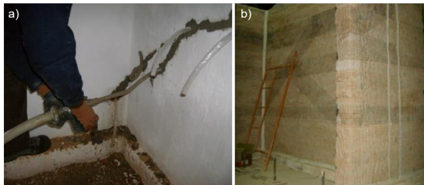
Figure 2: (a) Injection of hydraulic lime into the cracks; (b) application of polymer mesh (Figueiredo et al. 2013)
