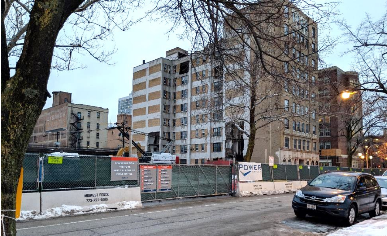
Figure 14. A demolition crew dismantles the apartment building at 6330 N. Winthrop Avenue (center), Chicago, February 20, 2019. Source: Author's collection.
