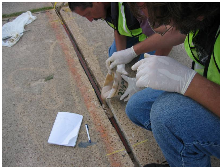
Fig. 33. Sensor bar installation: putting the metal bar in the slot and filling it with epoxy up to the top
