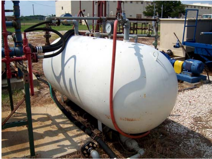
Fig. 62: Pressure Vessel for Compressed Air Storage
