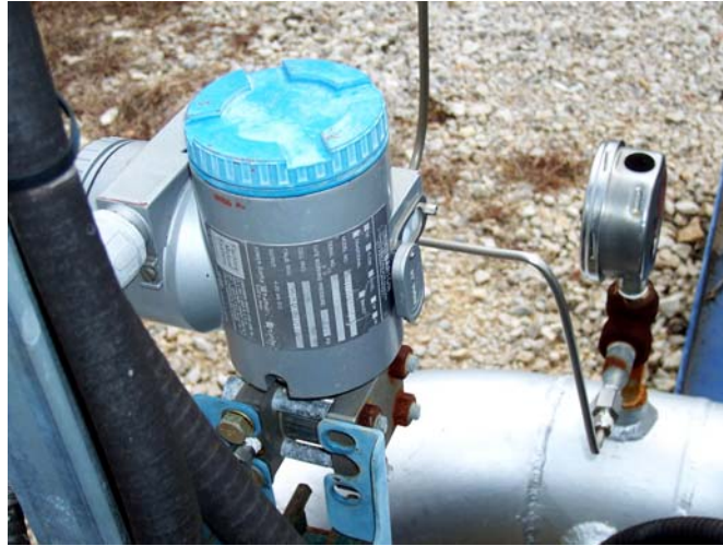
Fig. 68: Pressure Transmitter on Suction of Flowserve Twin-Screw Pump
