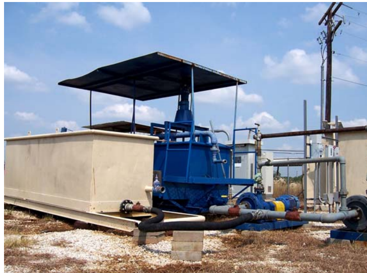
Fig. 61: Tanks and Feed Pumps
