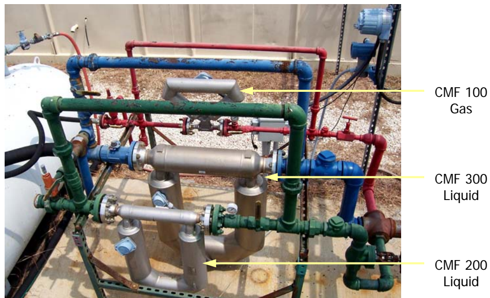
Fig. 64: Gas (Red Line), Water (Blue Line) and Oil (Green Line) Coriolis Meters
