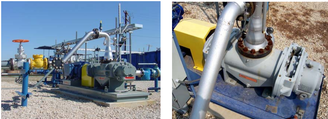
Fig. 36: Flowserve LSJIS Twin-Screw Pump at Texas A&M University Riverside Campus
