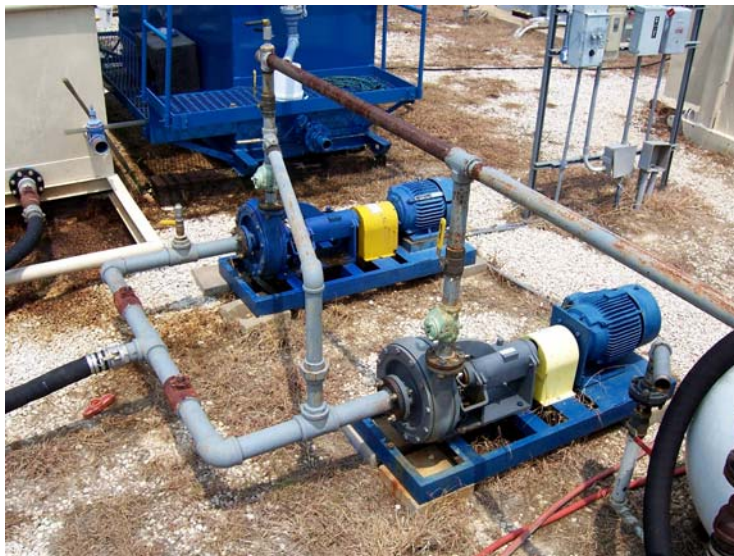
Fig. 63: Centrifugal Feed Pumps
