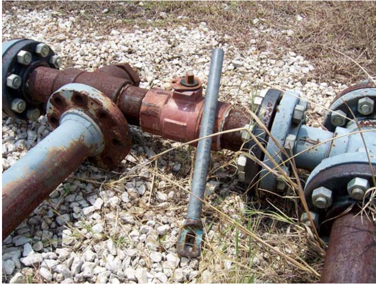
Fig. 75: Valve used to Buildup High Pressure on Discharge Side
