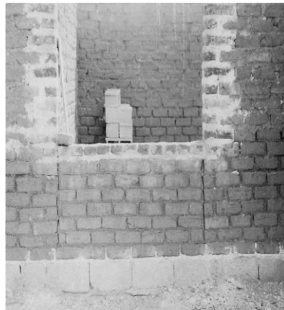
Figure 12: Fissure opening at the lower part of the wall, under the window
