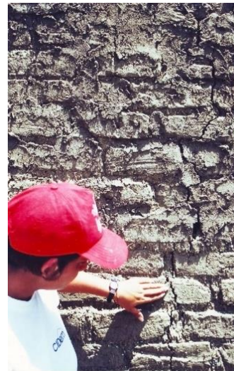
Figure 4: Cracks into wall without pillar
