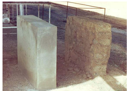
Figure 15: Difference between coated and uncoated walls
