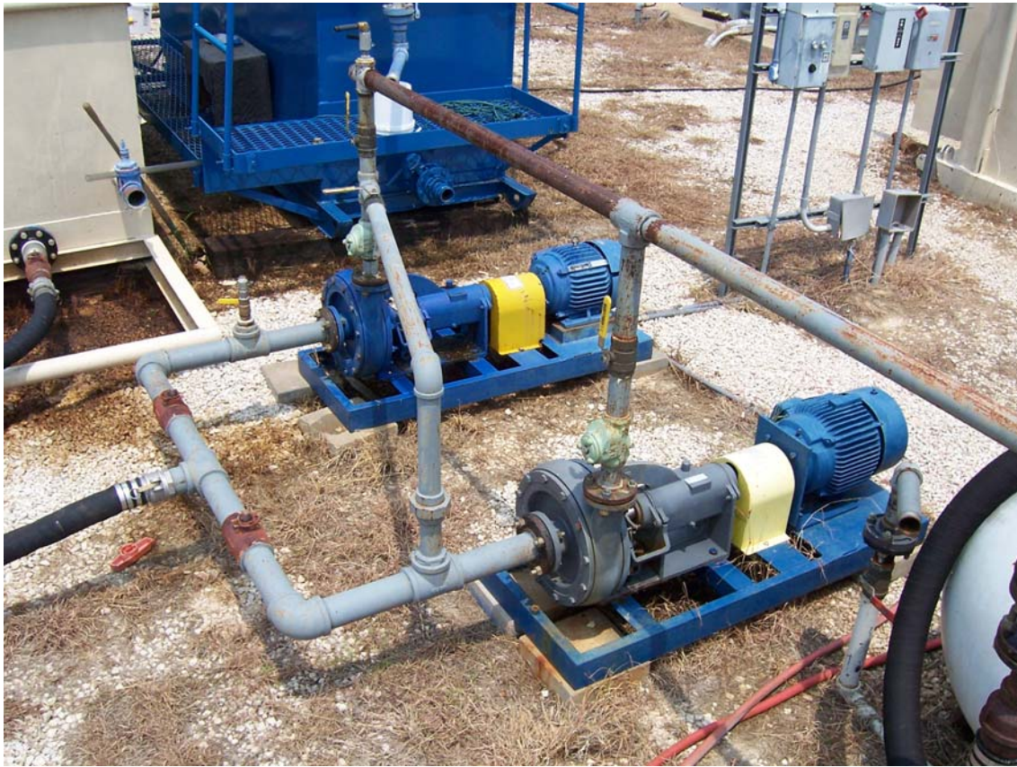
Fig. 4.4 – Centrifugal charging pumps.
