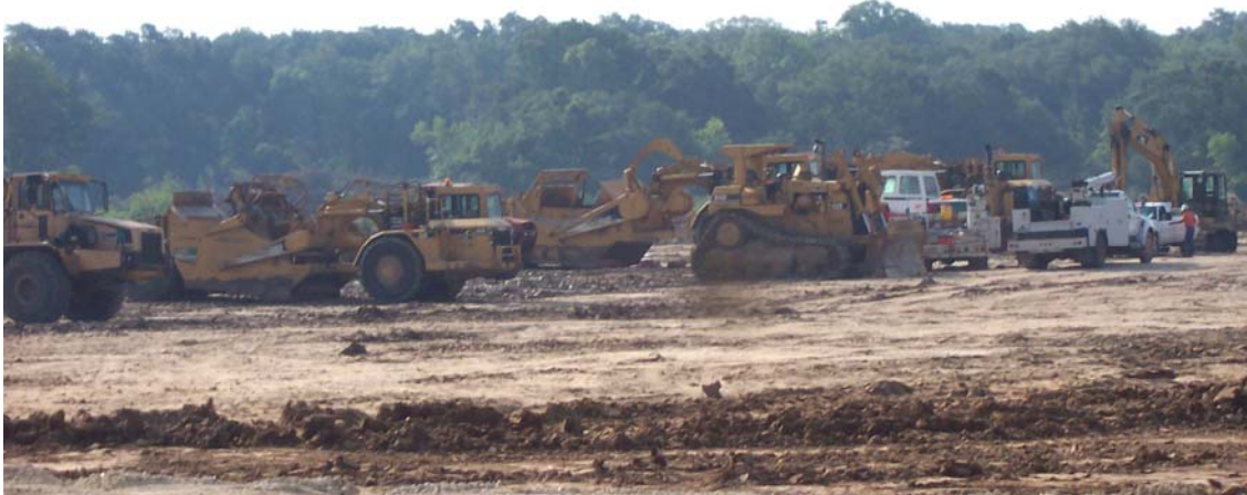
Figure 12. Equipment being Serviced on the Job Site
