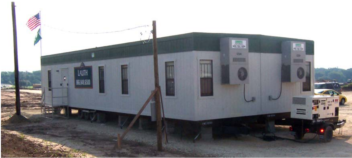
Figure 10. Photograph of the Construction Trailer, Service Drop and Generator
