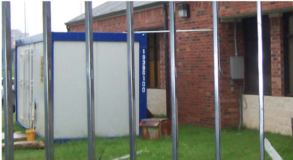
Figure 13. Electrical Service to the Construction Trailer and the Building under Construction for Project B
