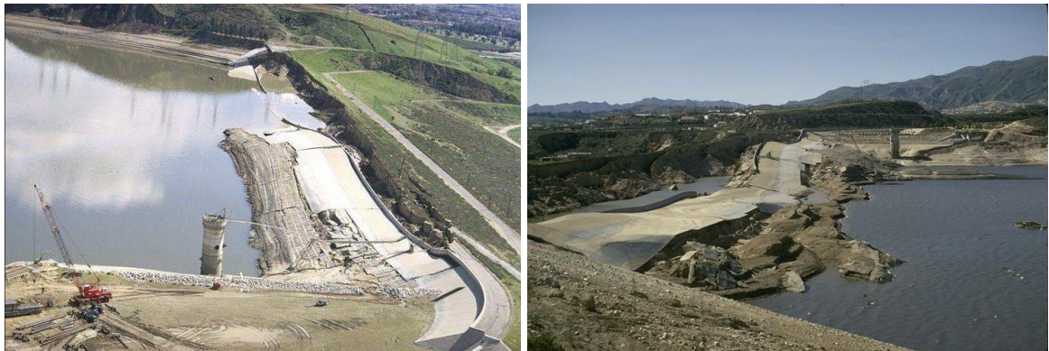
Fig. 5. Lower San Fernando Dam Collapse due to San Fernando Earthquake in 1971 (after NISEE 2016).
