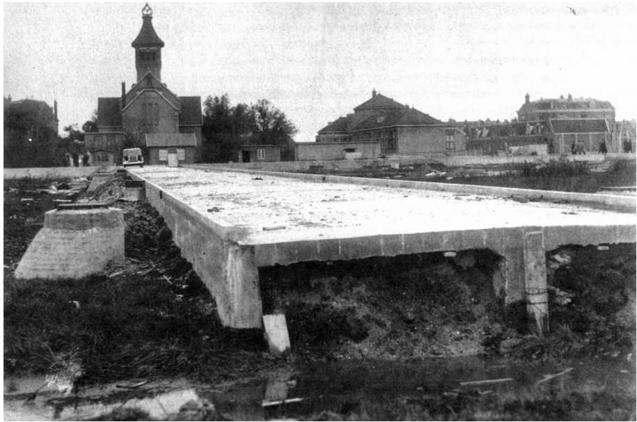
Figure 5a. The Paulus Emtinckweg (one of the roads built on sunken piles) under construction in 'De Nieuwe Buurt'. In the background is the crossing Burgemeester Van Tienenweg (built on sunken piles in 1934), behind which the back of the Sint Petrus Banden church can be seen (1910); on the right of the photograph, parallel to the Emtinckweg, are the Schoolstraat (constructed in 1934) with the Sint Petrus school and on the other side of the road, houses. Visible sticking out above the houses is the roof of the former town hall of Diemen (1882). (Photography: Jan de Boer, 1934) For details on the location of the streets, see Figure 6.
