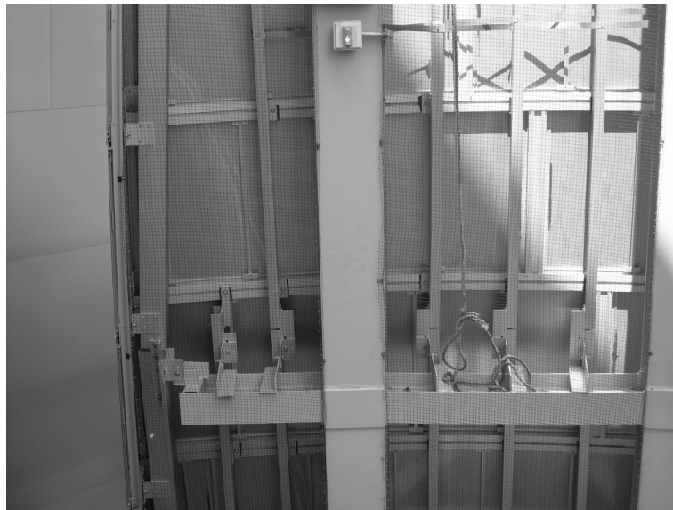
Fig.5.36 – The steel structure behind the metal skin at the Disney Hall. Top: A view of the steel structure behind the metal skin. Bottom: Close up view of the steel structure. (author).
