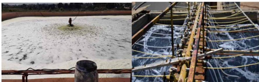
Figure 3 | Aerated biological units.
