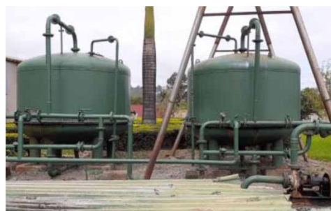
Figure 4 | Activated carbon filters.
