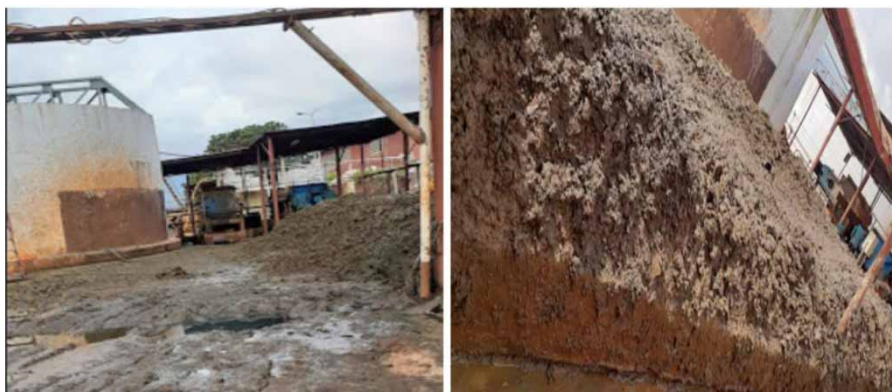
Figure 5 | Sludge produced after coagulation-flocculation process in primary clarifier.
