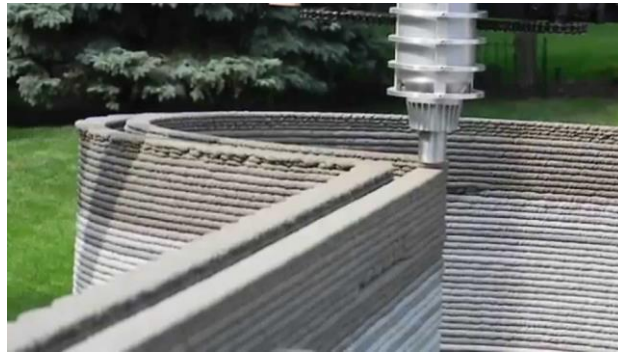
Figure 2. An example of how concrete should be laid in even layers without spreading
