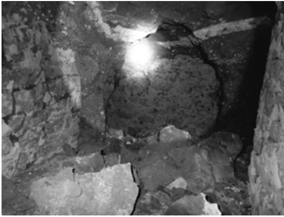
Photograph 4. Area of collapse in tunnel I-27 in September 2017.
