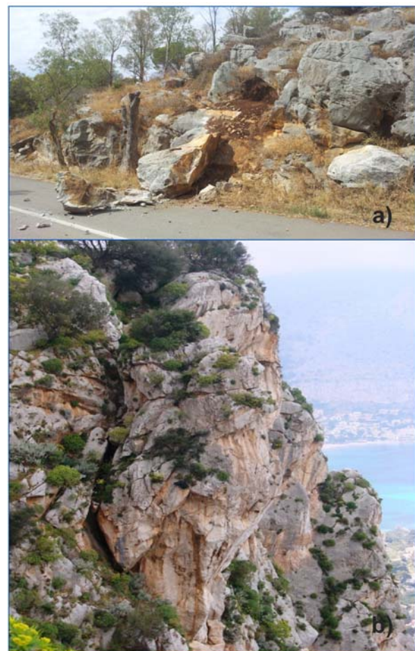
Figure 6. Example of a block-slide along the street leading to the Santuario of S. Rosalia. b. Unstable huge rock block in a rock wall affected by slide phenomena.
