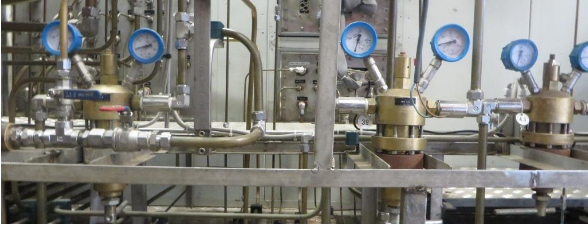
Figure 2-14. Pressure regulators with pairs of gauges.
