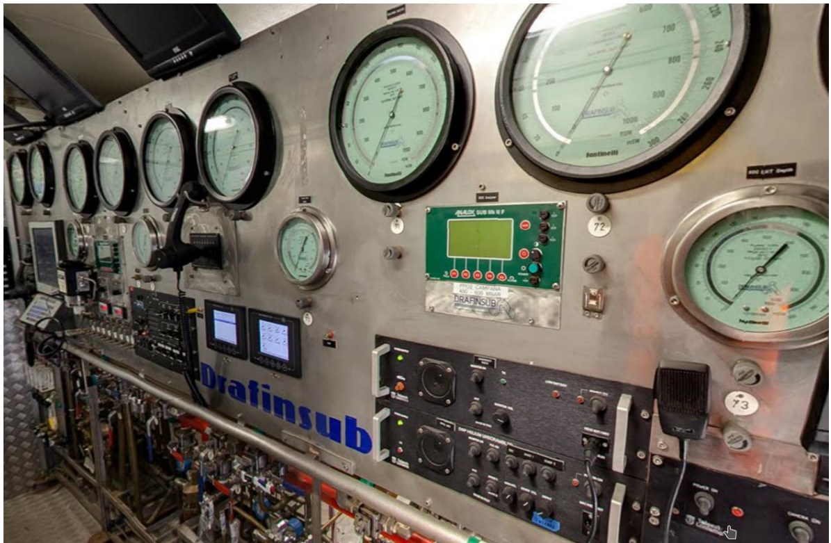
Figure 2-5. Typical control panel of a saturation diving plant.
