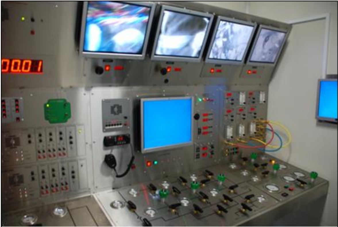
Figure 3-3. Saturation diving control panel of ADAS.
