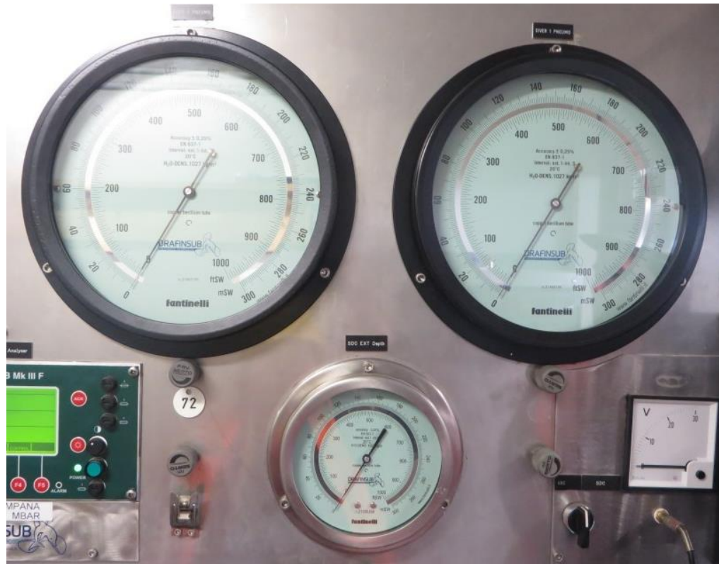
Figure 2-11. Pressure gauges in the control room.
