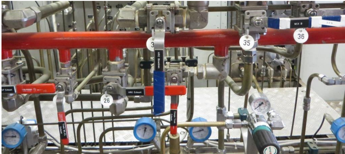
Figure 2-13. Gas pipes connected to the manifold (red) and corresponding valves.
